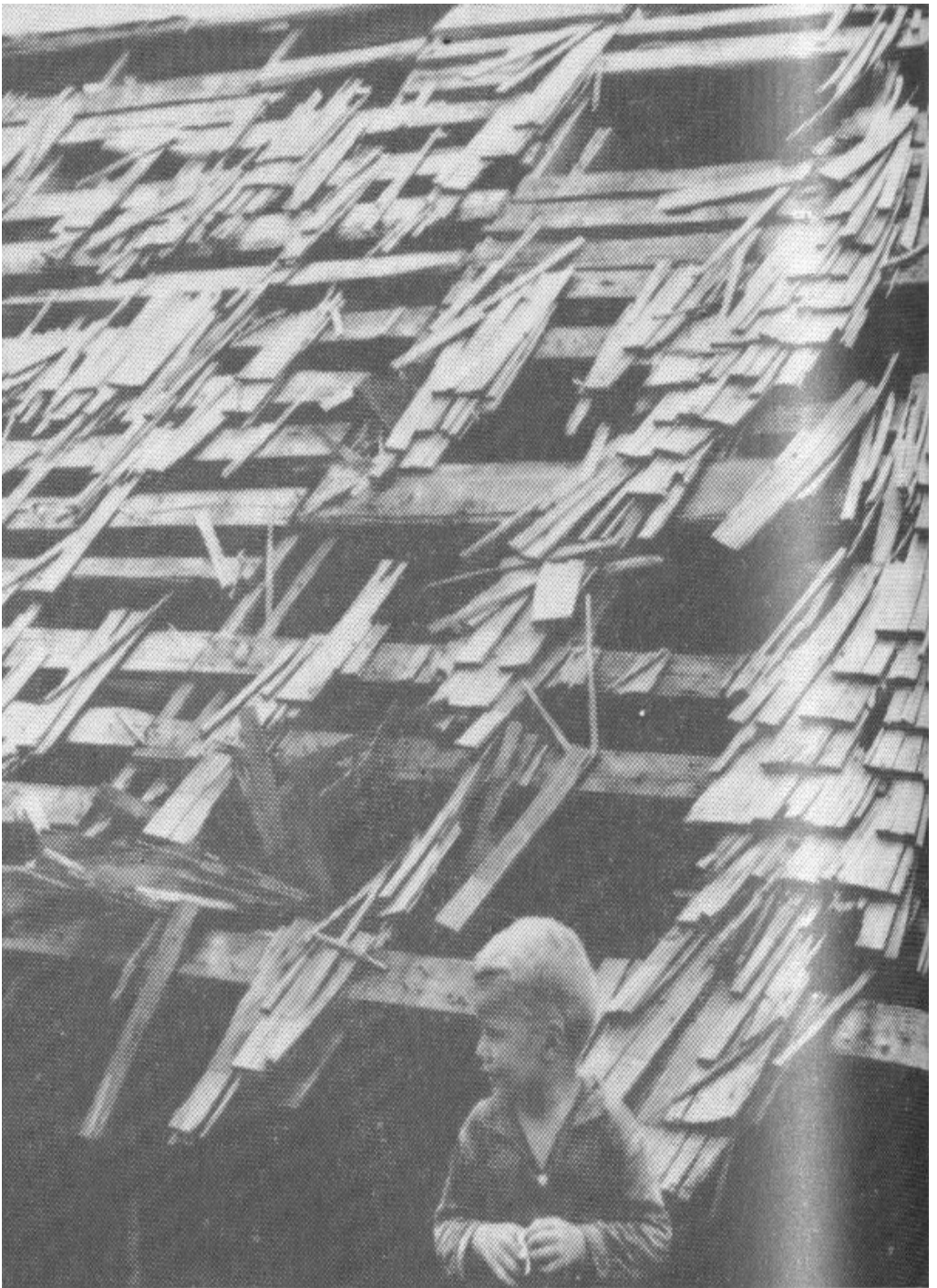
What hail can do to a shingle roof. Near Weatherford,
