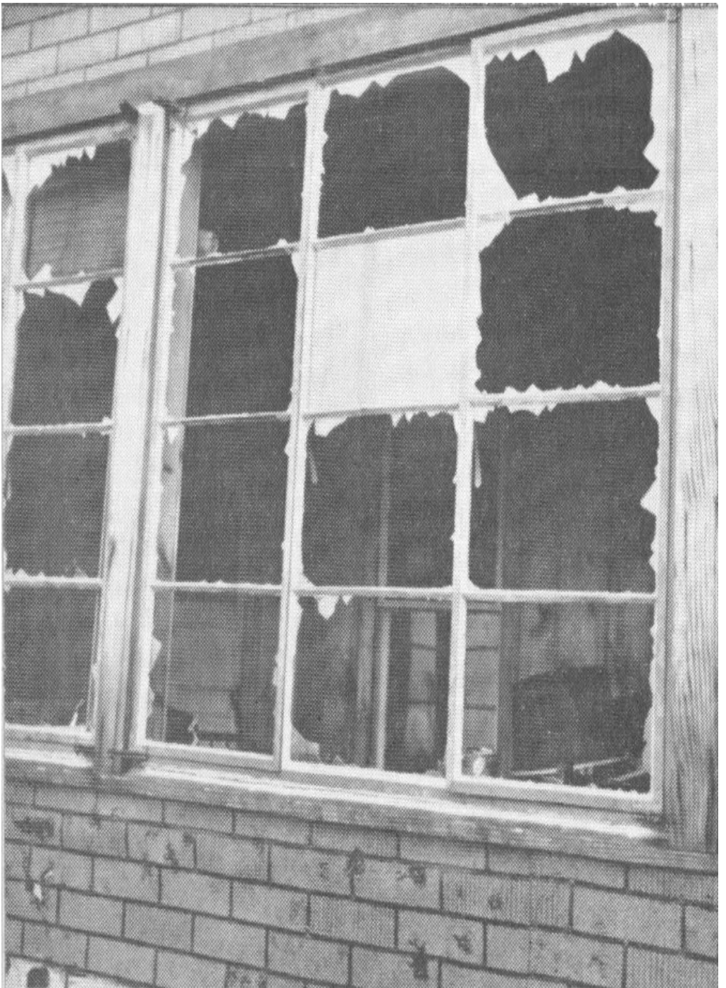
Windows after an Oklahoma hailstorm. This storm
